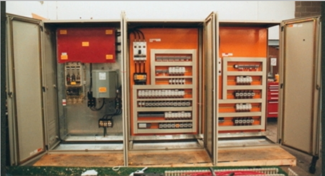
Recycling Plant - Power Distribution Control System
