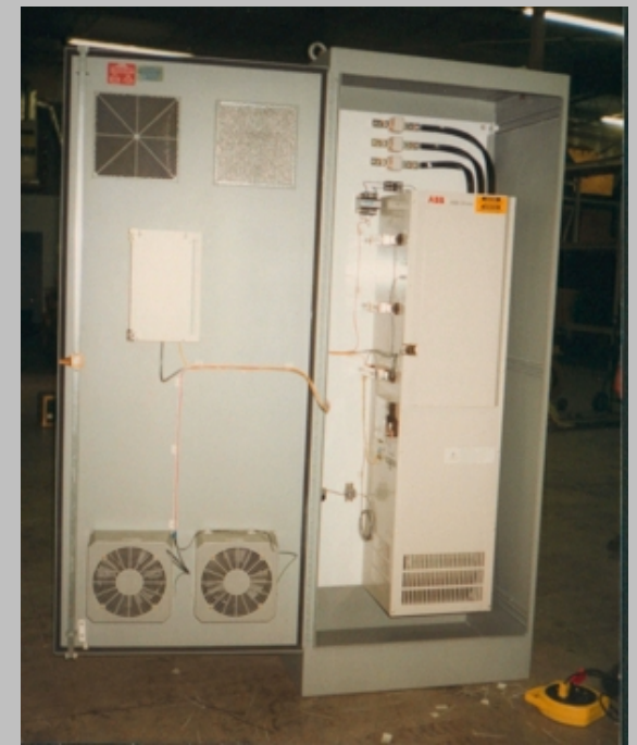
ABB - AC Drive Cabinet
