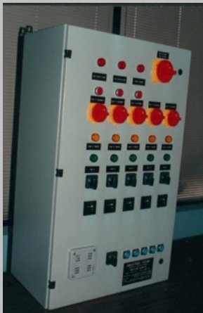
Custom U.L. Control Panels
