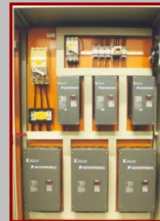
Motor Drive and Control Cabinets
