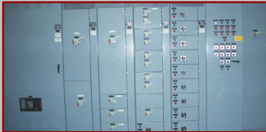
U.L. Motor Control Centers - 2000 AMPS
